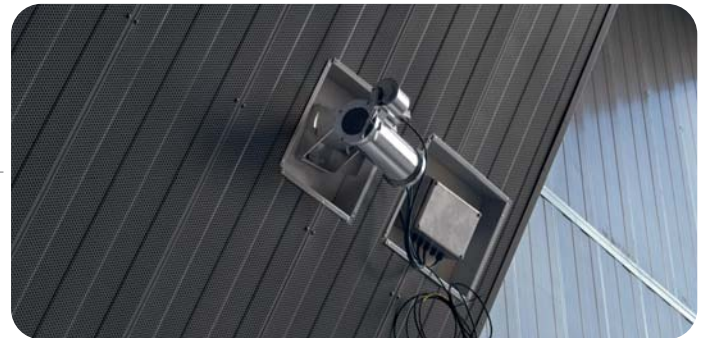
Special cameras automatically detect dangerous situations.
